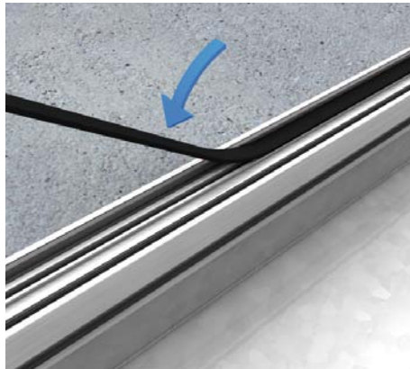
38 | Duct system for wet-cleaned linoleum floors Glue the rubber seal (UGDB15-R300 1.8) onto the side profile in longitudinal direction, covering the entire area of the duct.
